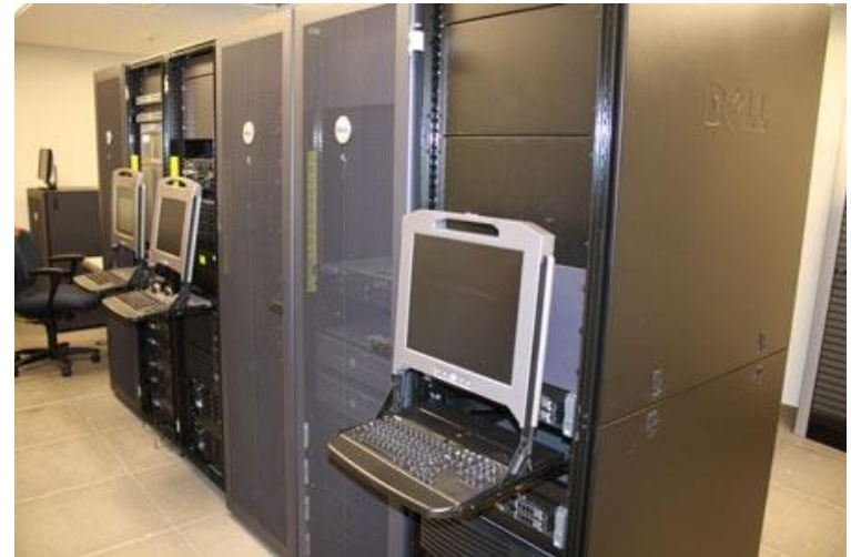
AFIS installation at Michigan State Police facility. This system was first installed in 1989; the database has 3.2 million tenprint cards and performs 700,000 searches each year
